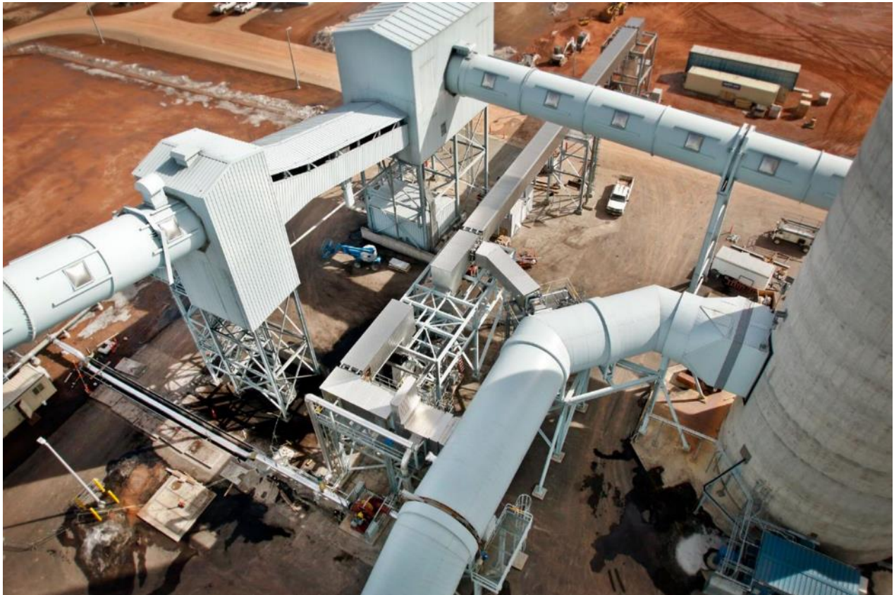
Fig. 3 – Overview of ITC connection to Dry Fork Station
