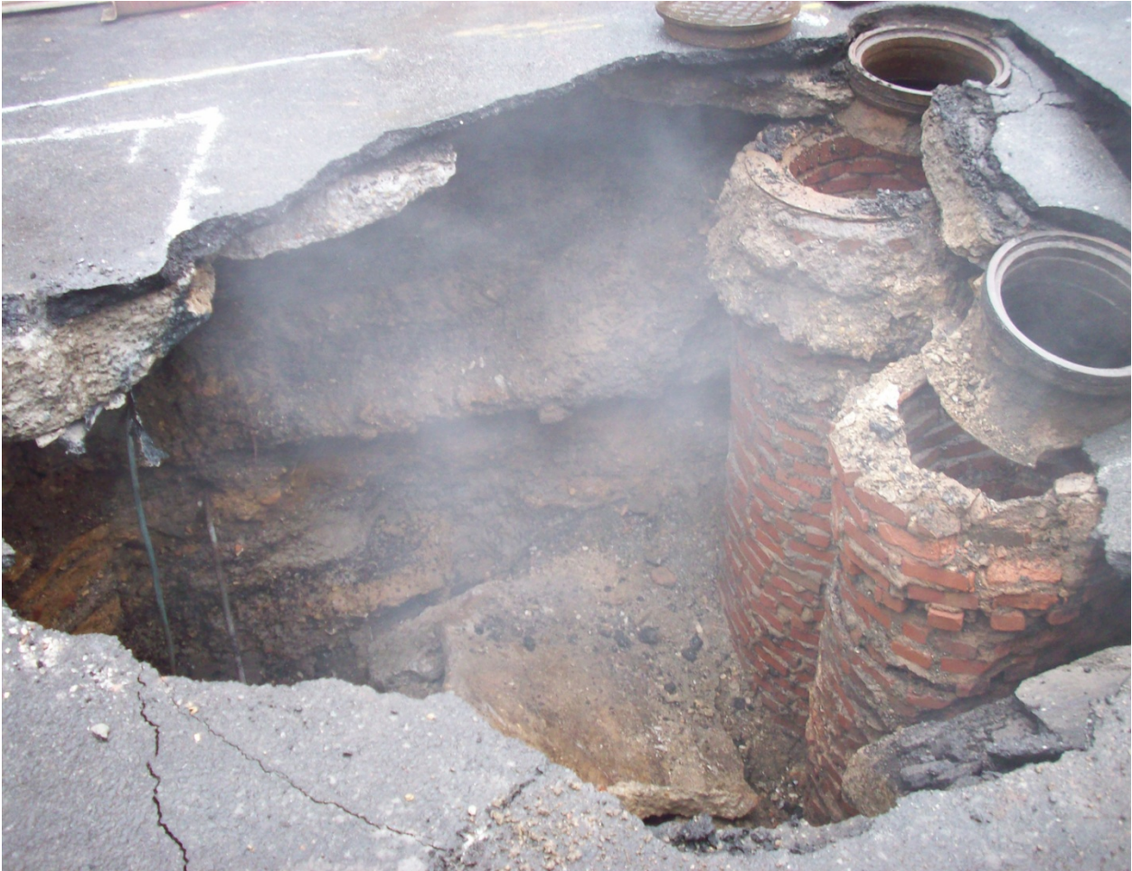
Damaged Sewer – Spring Place NW, December 2009
