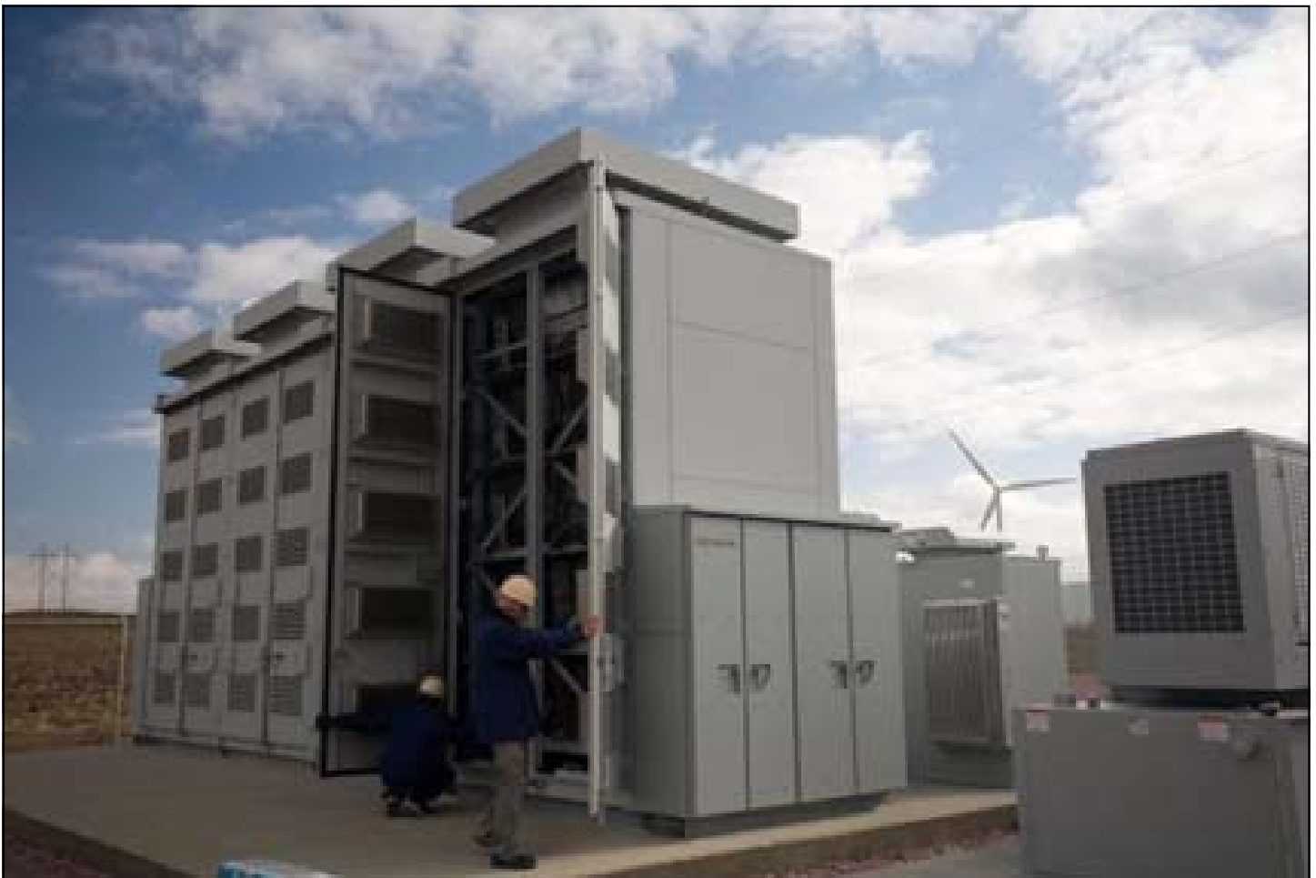
Xcel Energy wind-to-battery project, Minnesota
