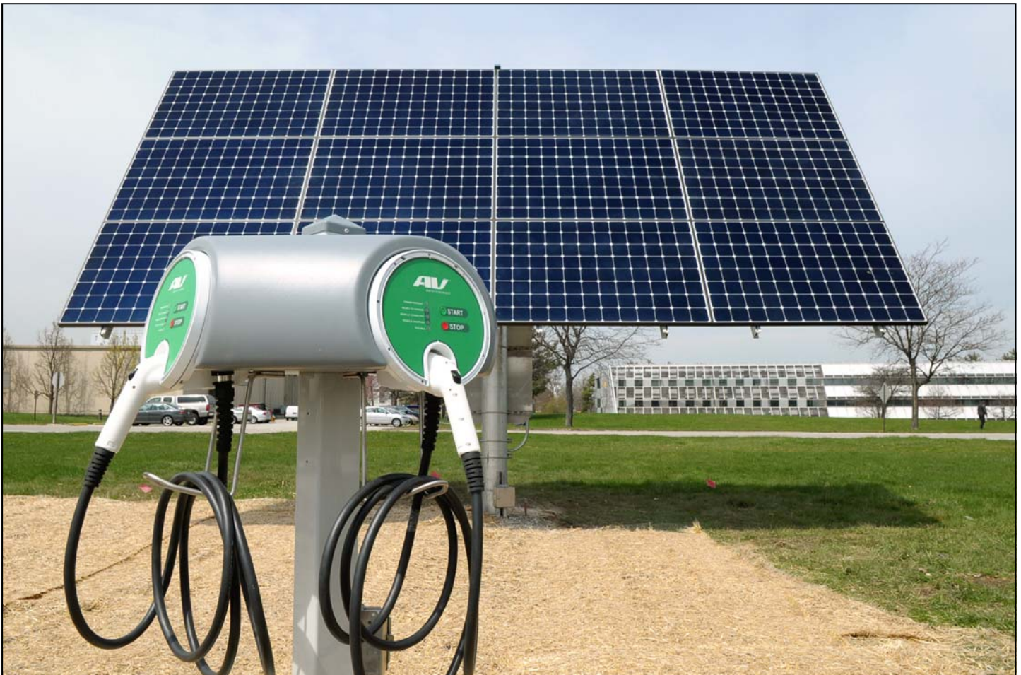
Solar powered electric vehicle charging station at Argonne National Laboratory (ANL)
