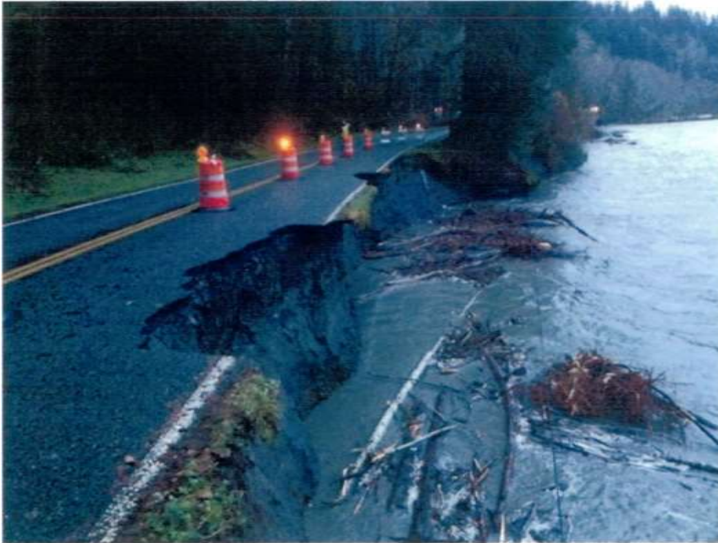
Damage to the Upper Hoh Road, November 2014
