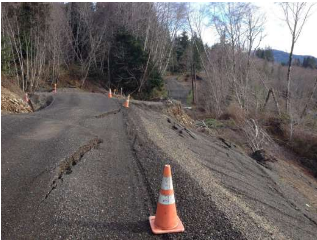
Damage to Undi Road (Landslide), 2015
